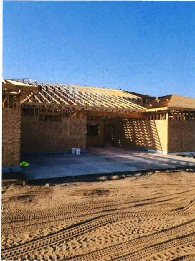
Construction begins on ABLE, Inc.'s transformative intermediate care facility in Hettinger. Photo courtesy of ABLE, Inc.
